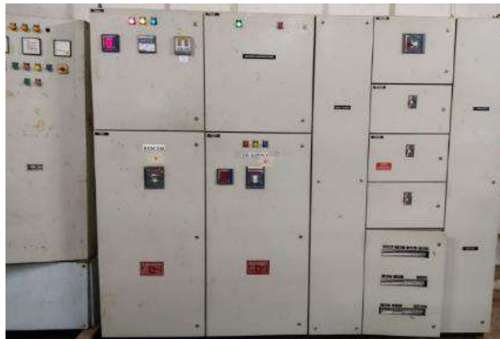
Figure 5-2: Electrical Panel Room
