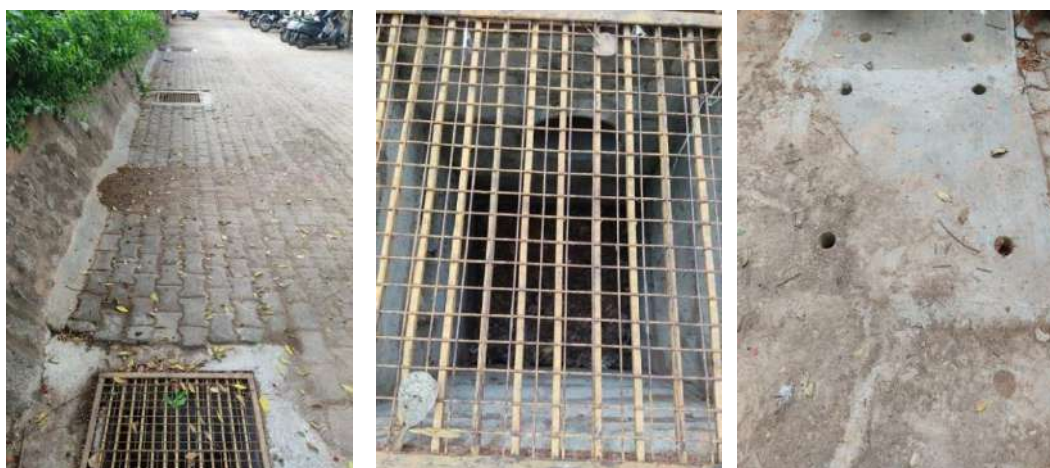
Figure 4-10: Percolation pits for rain water harvesting
