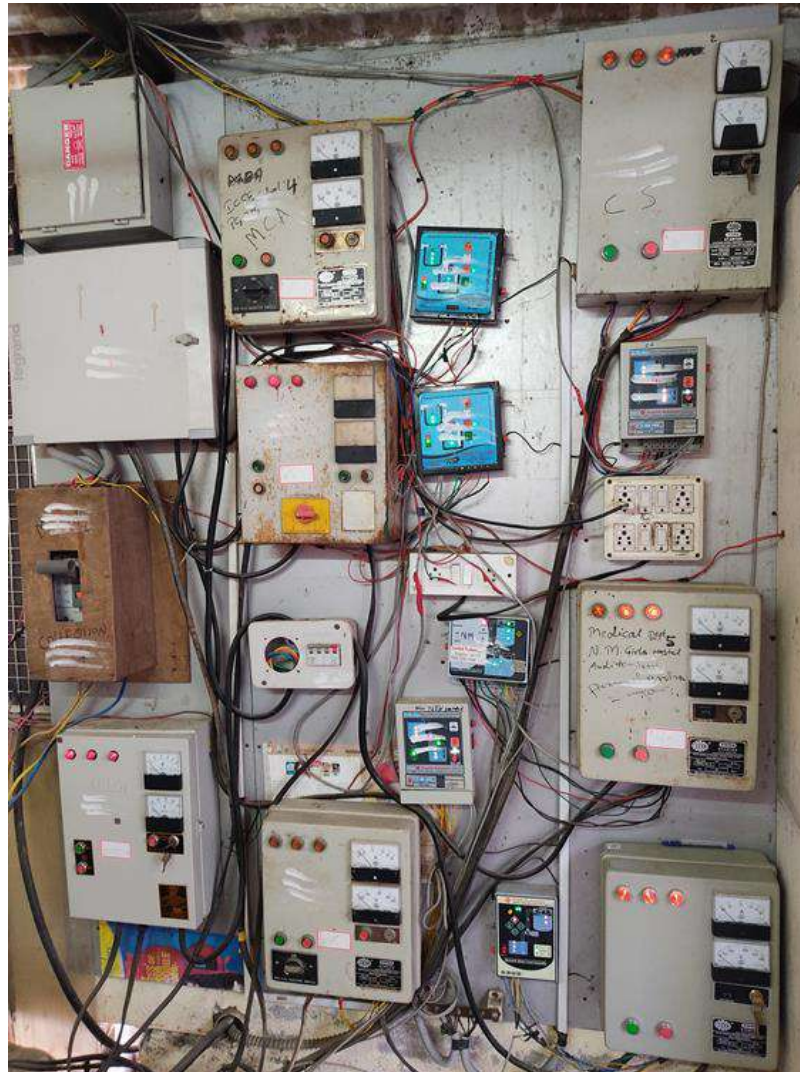
Figure 4-2: Pump house water controllers and meters
