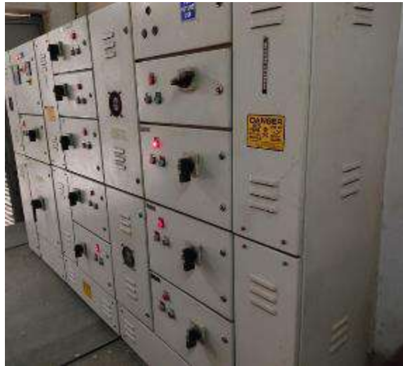
Figure 5-3: Capacitor Bank Panel
