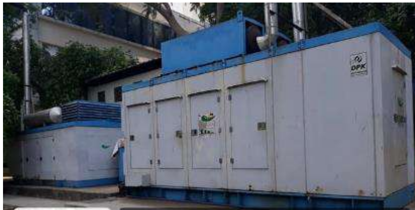
Figure 5-4: 400kVA and 250 kVA Diesel Generator (DG) set
