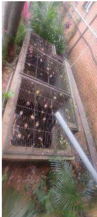
Figure 4-23: RWH sump near dental blocks
