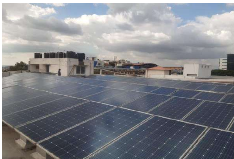
Figure 5-6: Solar rooftop PV system
