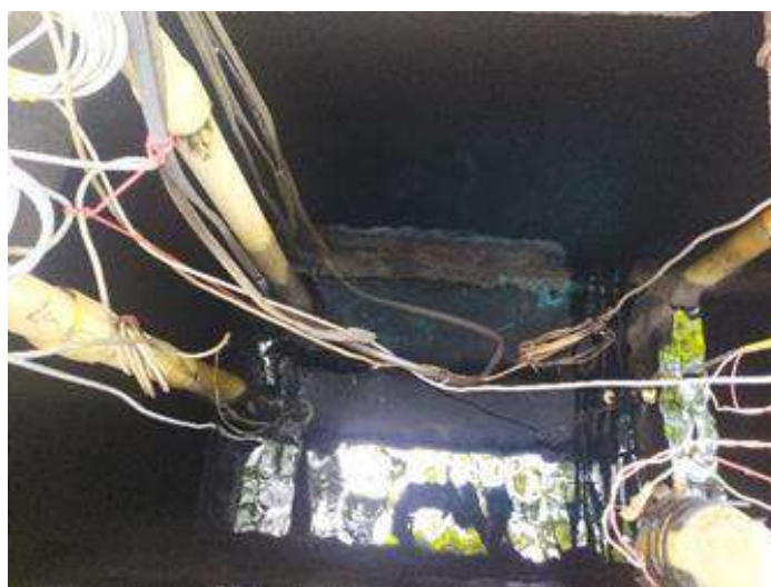
Figure 4-1: Raw water sump level controller
