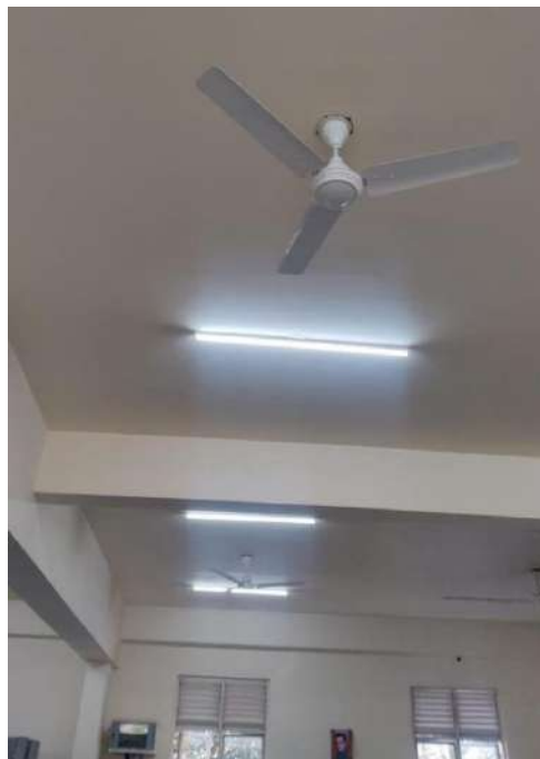
Figure 5-13: LED lights in Classrooms, Labs, and Corridors
