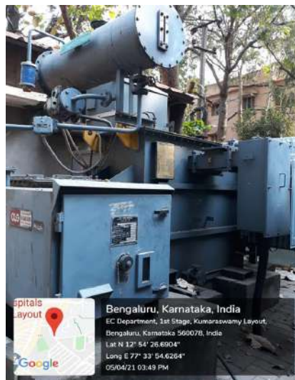
Figure 5-1: Transformer unit Installed in the campus
