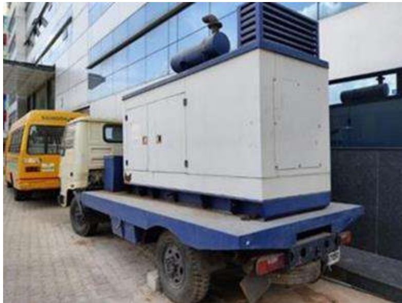
Figure 5-5: Mobile Diesel Generator (DG) set
