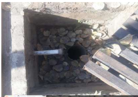
Figure 4-9: Rain water harvesting Percolation pit
