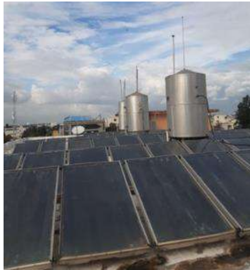
Figure 4-13: Hot water system in hostel
