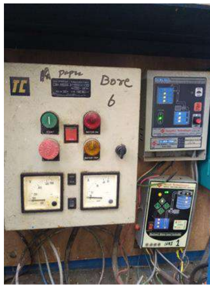
Figure 4-4: Bore-well pump panel and level controller switch
