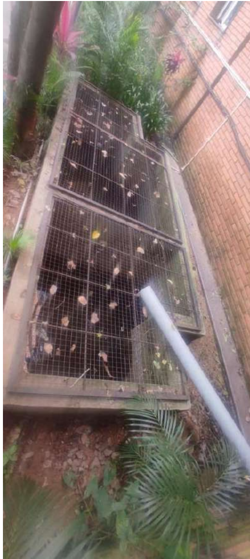
Figure 4-11: RWH sump near dental blocks
